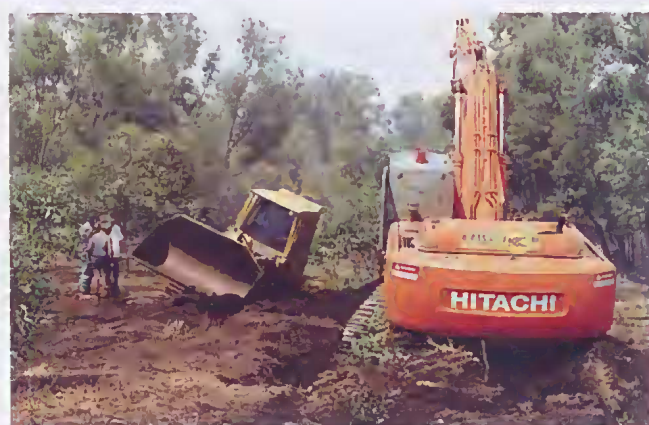
Figure 3. Equipment bogged in the peat.
